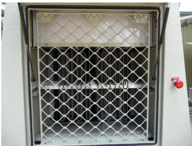
Fig. 4. Front view of the HPTX-80 with the door open showing the dummy load protected by an aluminum mesh screen.
