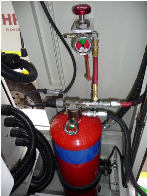
Fig. 12. The fire suppression control system located in the right side of the electrical compartment.
