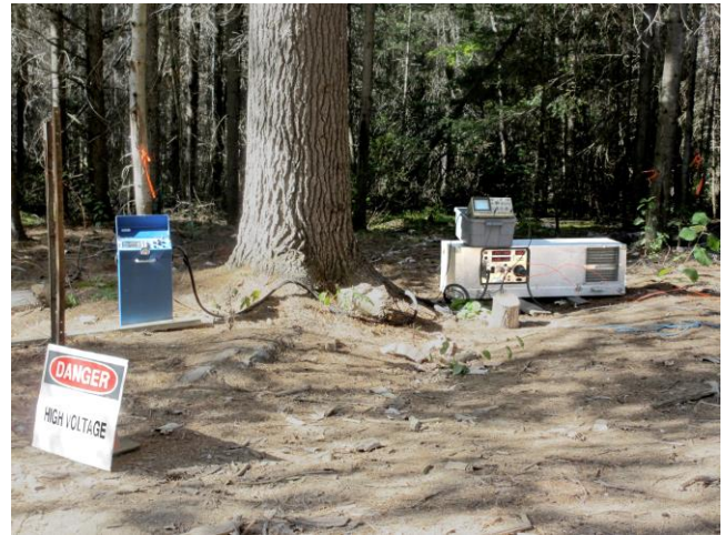
Figure 5: UTEM 4 transmitter setup. The control unit on the left is connected to the 1.4m long power mainframe unit by a cable of multiple optical fibres. The 11kW power generator is off the photograph.
